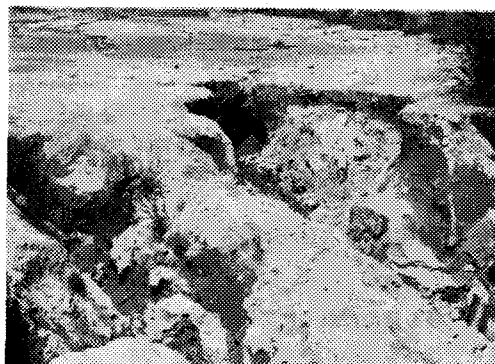
Fig-6 Landslide of the field slope
